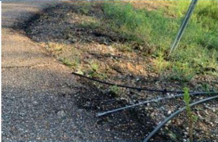
Do not cut lines. It is faster to repair than to replace damaged lines.
