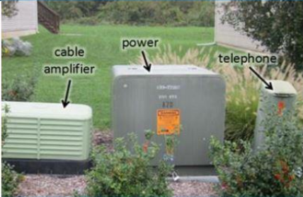
Do not pile debris on or near utility pedestals.
